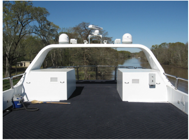
The two air handler on Sky Deck are enclosed in the weathertight cabinets
