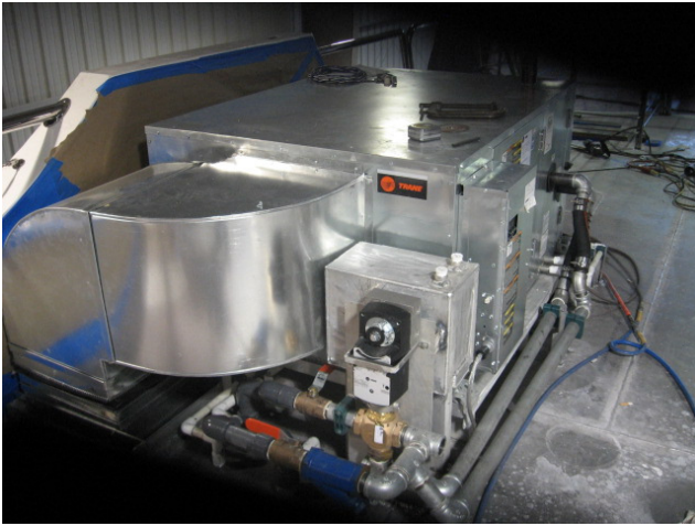
One of the air handlers, shown during installation on the Sky Deck
